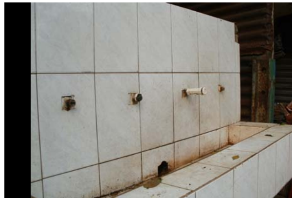
Broken water taps
