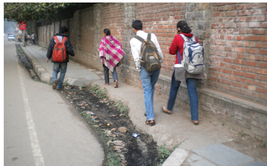
Broken/ Narrow Pavements in New Delhi
