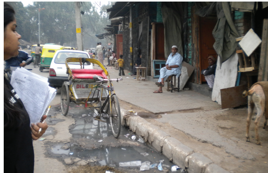
Condition of pavements (Ajmeri Gate – Delhi Gate site)
