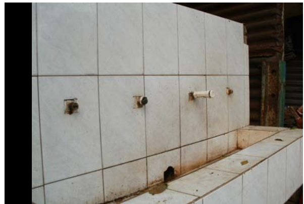
Broken water taps
